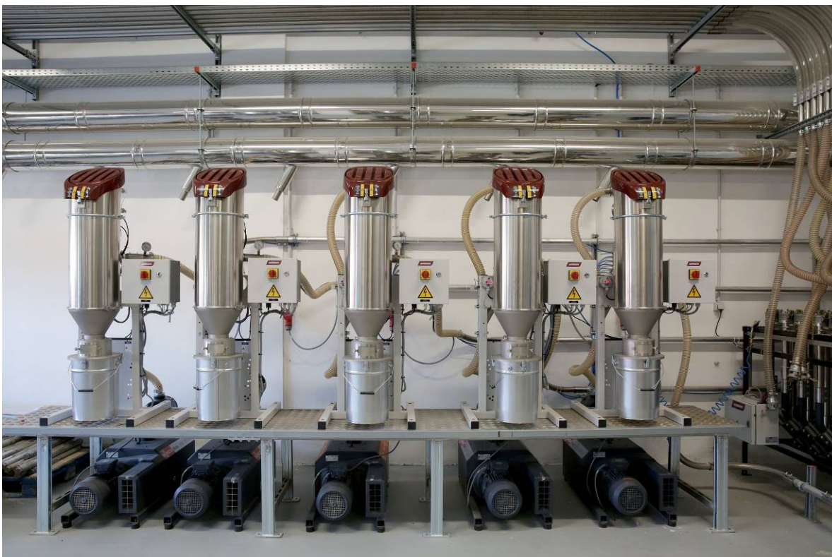
Fig. 4: WITTMANN Central Conveying System (Photo: WITTMANN BATTENFELD Romania)
