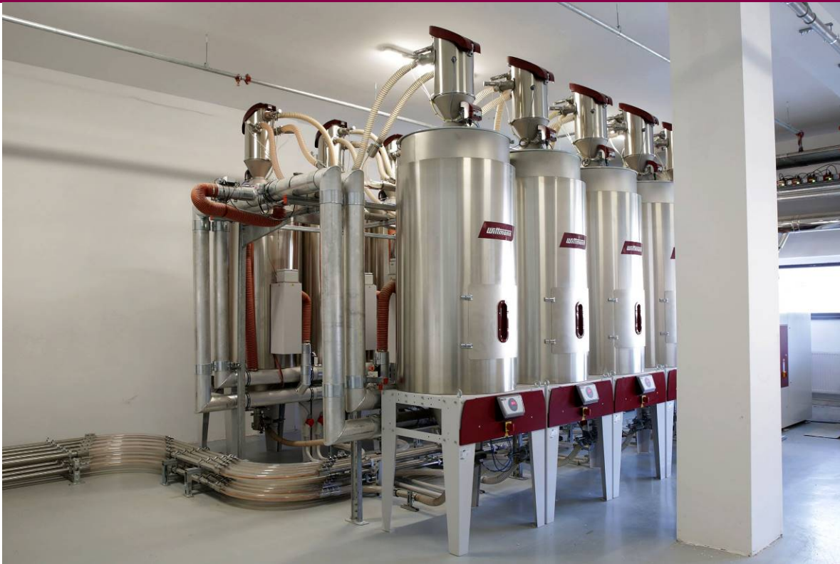
Fig. 5: WITTMANN Central Conveying and Drying System (Photo: WITTMANN BATTENFELD Romania)
