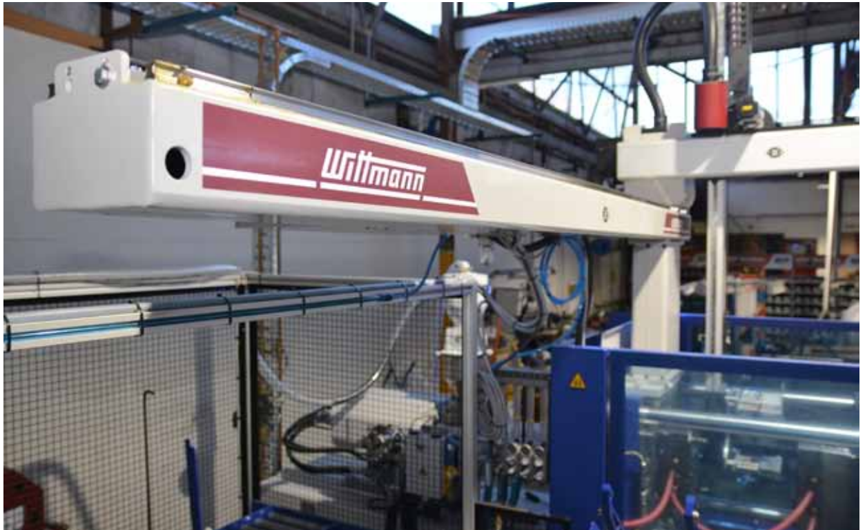
View of an injection molding working cell from the WITTMANN Group, consisting of a WITTMANN BATTENFELD injection molding machine and a WITTMANN robot, installed at MtM Pty Ltd. in Melbourne, Australia.
