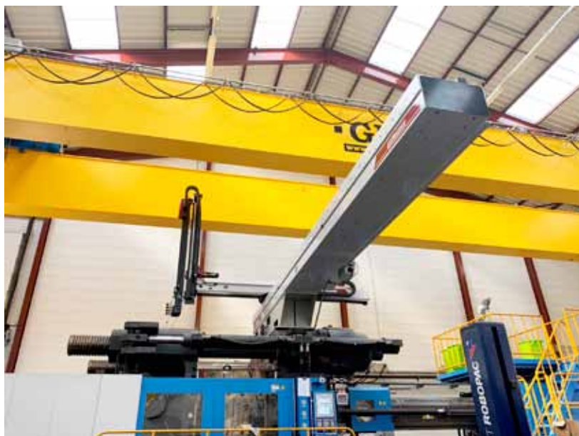
WITTMANN W873XL robot, photographed during the installation phase at BELLI in Bellignat, France.
